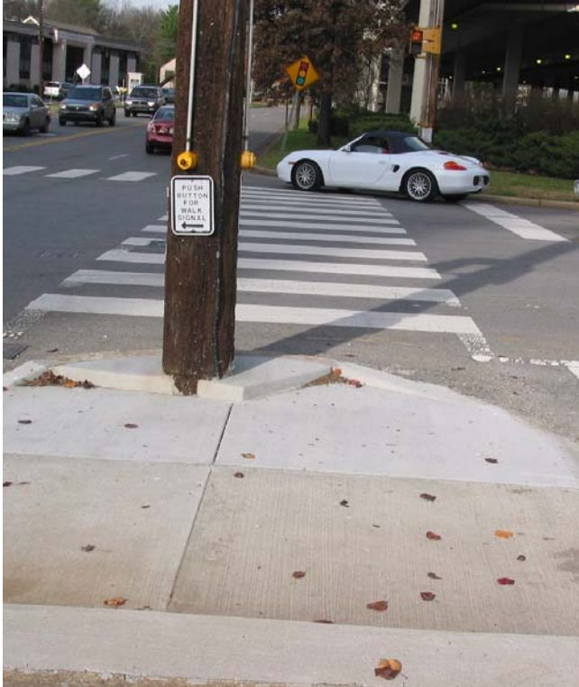
Metro Public Works improved this curb ramp near the senior center on Abbot Martin by making it ADA compliant and providing easier access to the pedestrian push button.
